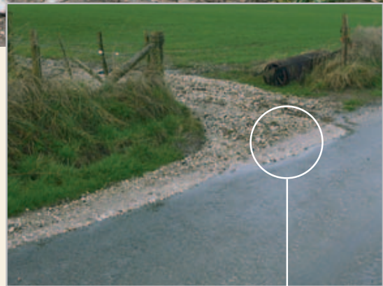
Runoff onto adjacent road
