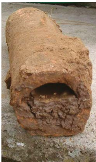
Figure 22. Silted clay drain
